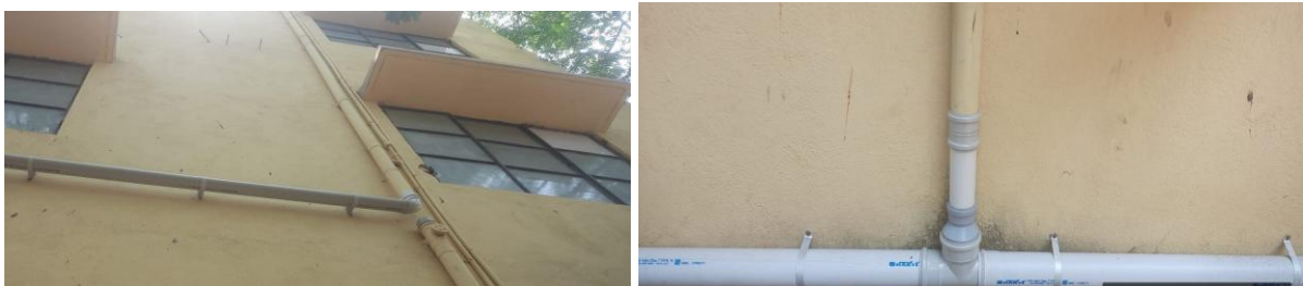
Rainwater collection pipe for Ground water recharging:
