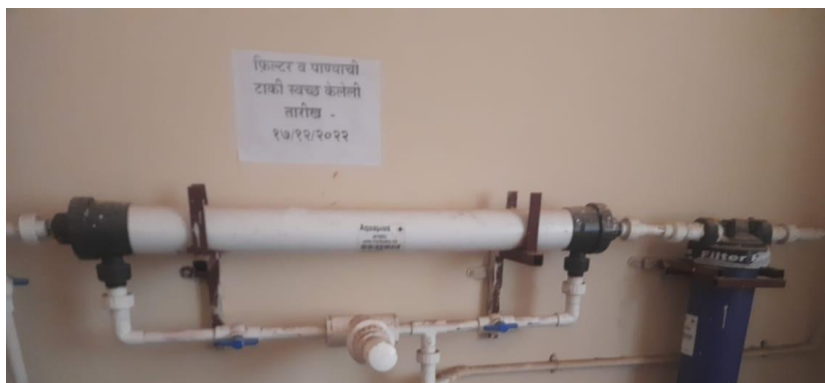
Advanced water filter unit
