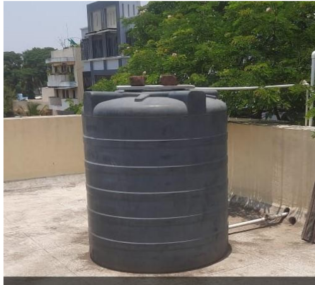
Collection tank for water storage
